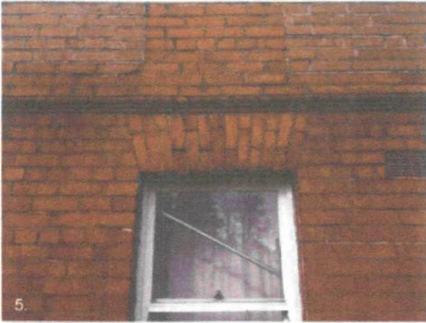
EXTERNAL FACADE – TYPICAL AREAS TO BE REPAIRED
